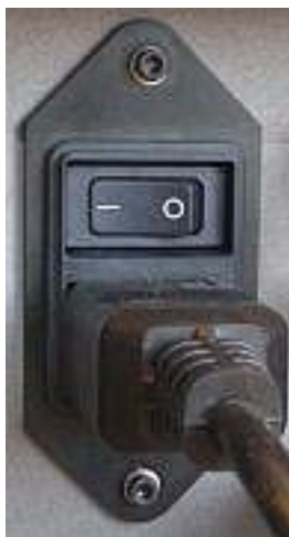
Figure 6-2: Main power switch and cable
